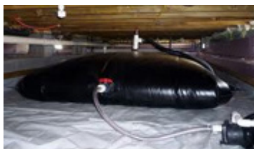
Example of a rain bladder installed under subfloor
