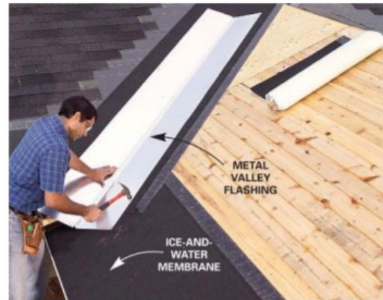
The installation of flashing in the new valley is shown. Note that existing shingles have been removed and ice and water barrier has been applied.
