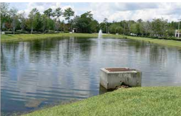
A typical wet pond and outlet control structure
