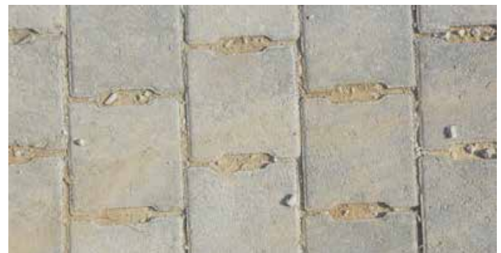
Clean permeable pavers (top) versus clogged (bottom)
