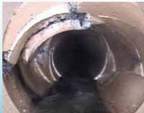
DAMAGED LAWRENCE SEWER PIPE
