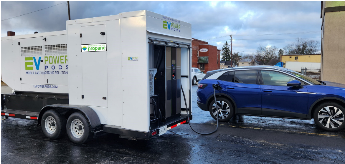
FIGURE 22. EV BEING CHARGED BY EV POWER POD
