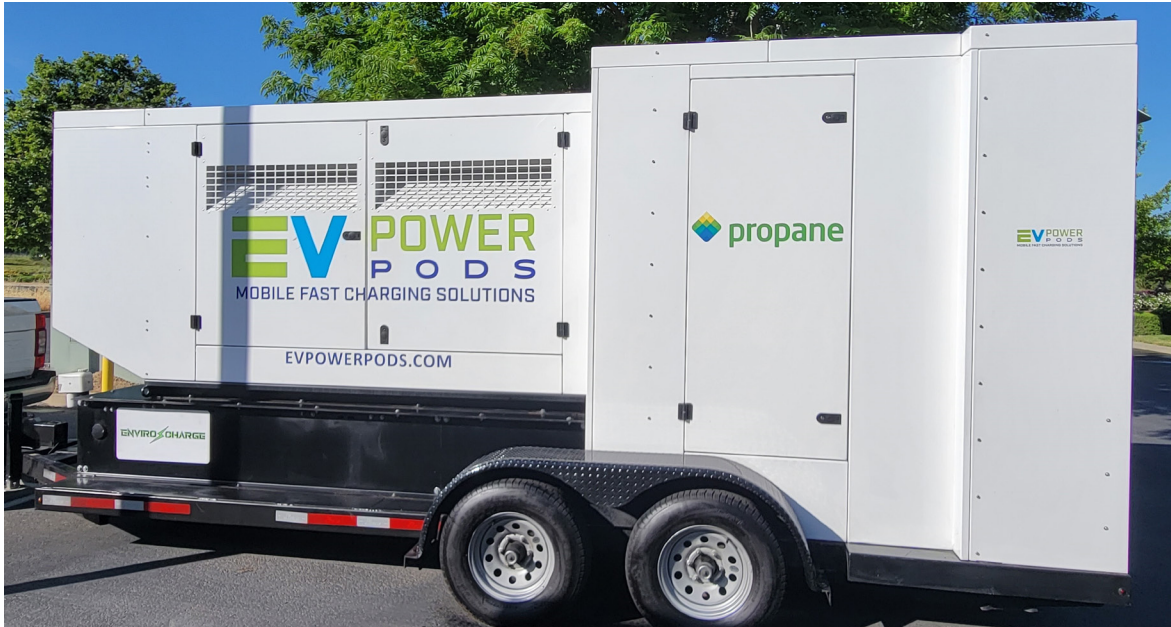
FIGURE 21. EV POWER POD TRAILER
